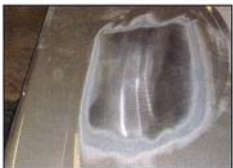
4 Remove the paint from the repair site and identify the highest spot. This will be the site of your first shrink. After making your first shrink and cooling, the next highest spot will be the site of your next shrink, and so on.
