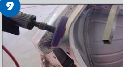
9 Remove all sealant and caulking to expose the resistance spot welds where the quarter panel is attached to the rear body panel.
