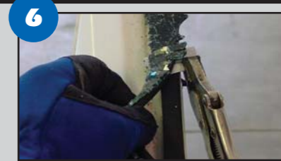
6 Cut out the urethane bead and broken glass to expose the rear glass pinchweld.
