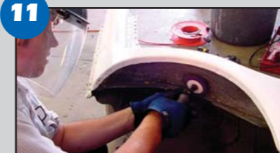
11 Remove the undercoating from the lip where the inner and outer wheelhouse panels are attached.
